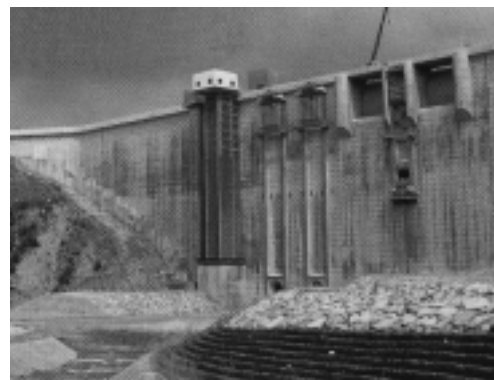
Photo 2 Hattabara Dam selective water intake facilities (1994) Telescopic cylinder gate to select warm or clean water
